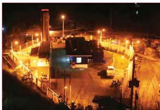
Biogas plant at night, powered by electricity from landfill gas, Quezon City, Philippines. The project is in receipt of carbon credits
