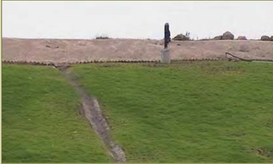
Gas venting pipe on waste dump
